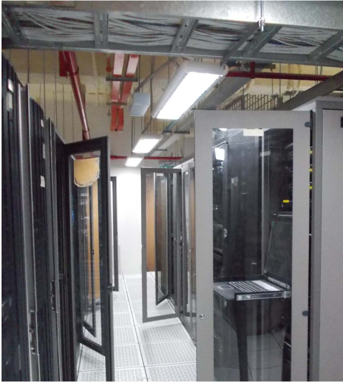
T6 lights in all server farm corridors.
