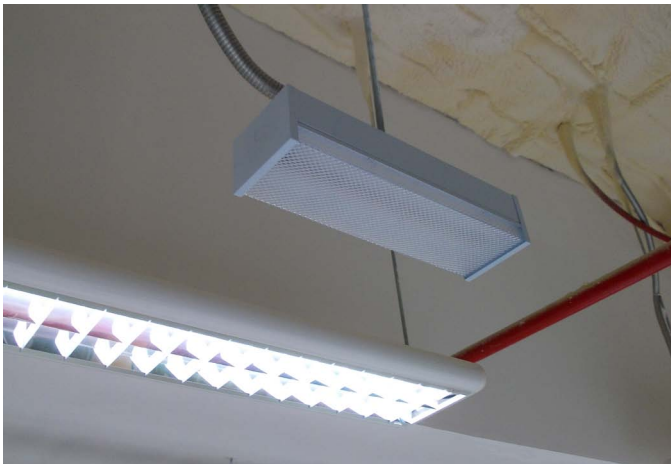
LED lights for all emergency lights.
