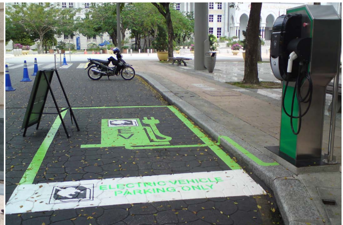
Temporary charging station is provided within the PJC complex area.
