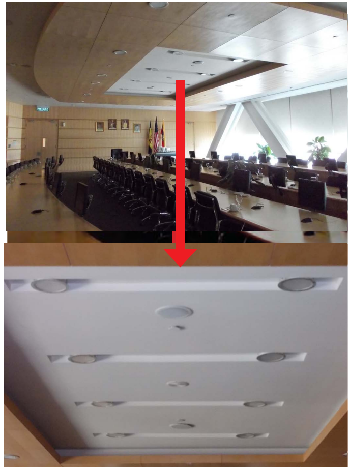
Tanjung Meeting Room which has been refitted with LED lights.
