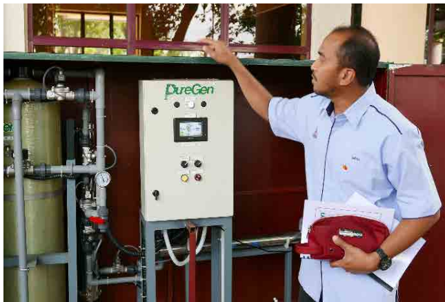
Rainwater collection and reuse system (SPAHS) at Surau Nur Ehsan, Petaling Jaya City Council headquarters
