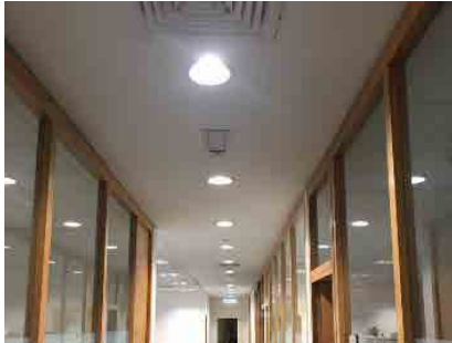
LED down light installed at the corridors.
