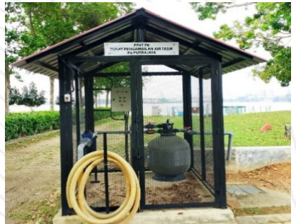
Lake water intake station at the Putrajaya Water Sports Complex, Precinct 6
