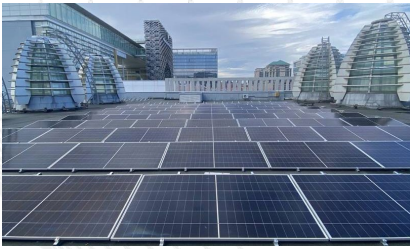
Solar photovoltaic at Putrajaya Corporation Complex, Precinct 3
