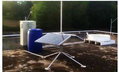
Portable Rain Monitoring System (WMS) at Putrajaya Sentral, Precinct 7
