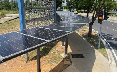
Solar photovoltaic covered pedestrian walkways at MRT Putrajaya Sentral, P7 – Pangsapuri Putra Harmoni, P9
