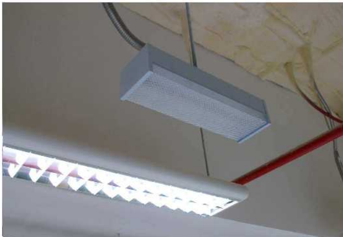
LED lights for all emergency lights.
