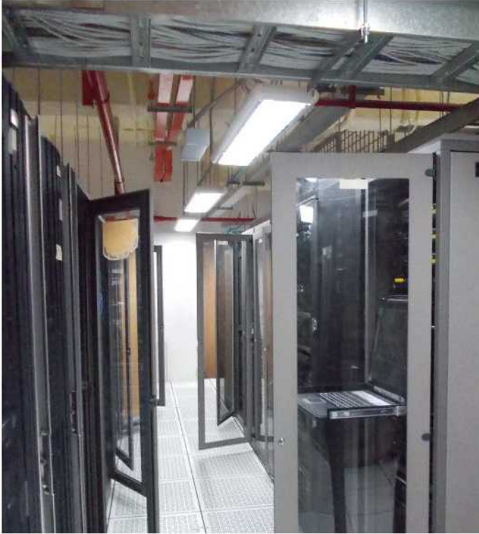
T6 lights in all server farm corridors.
