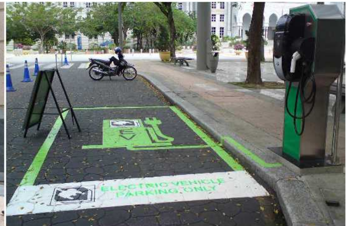
Temporary charging station is provided within the PJC complex area.
