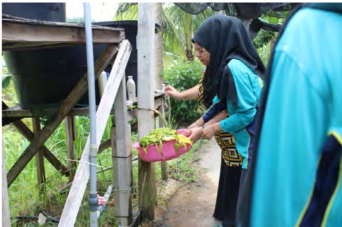
Rainwater harvesting facility is provided at the composting site.
