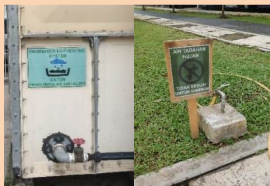
Rainwater harvesting systems
