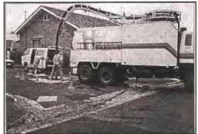
Figure 6.16 Removal of trapped material in the CDS device using a vacuum truck (ref. Allison et al, 1997)
