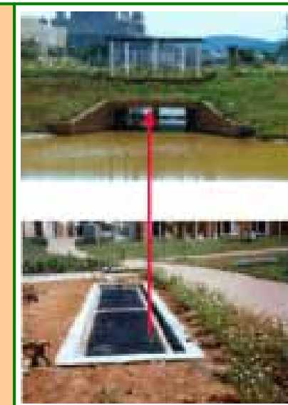
Gross pollutant trap to treat the water flowing into the lake
